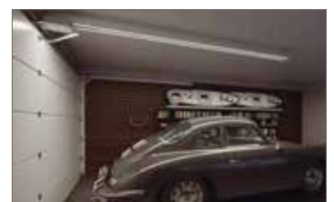
Installations on spring shaft/cross beam
